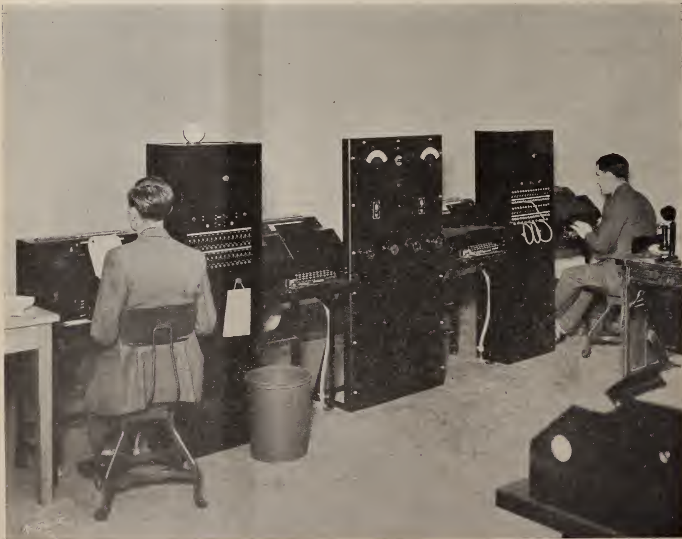
Central Teletype Broadcasting Equipment
